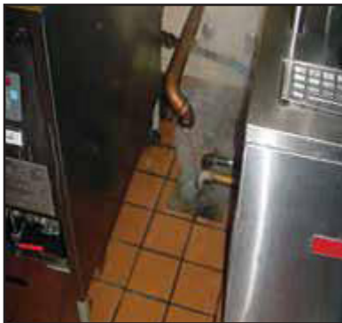
Drain pipe splashing excessive moisture
